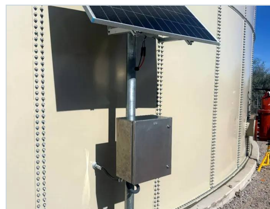
POST-MOUNTED UNIT – 550,000 GAL BOLTED TANK, ELOY AZ
