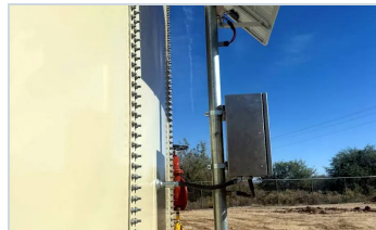
Panel and cabinet on the tank shell — Eloy AZ
