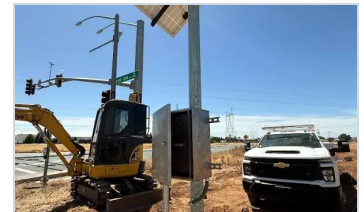
Pole-mounted, new force main — Elk Grove CA
